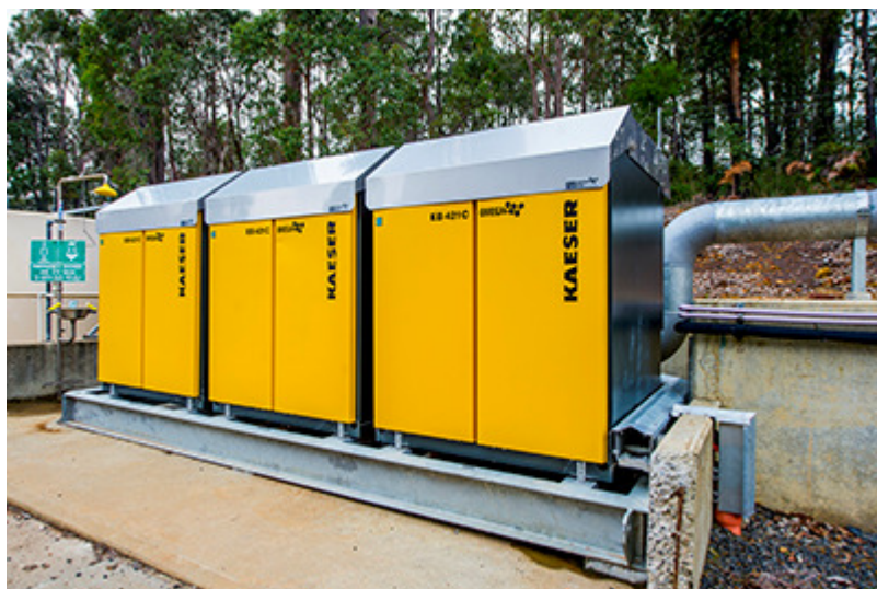
Caption: Three Kaeser Compact EBC series blower systems are being used for aeration at the Collie WWTP
