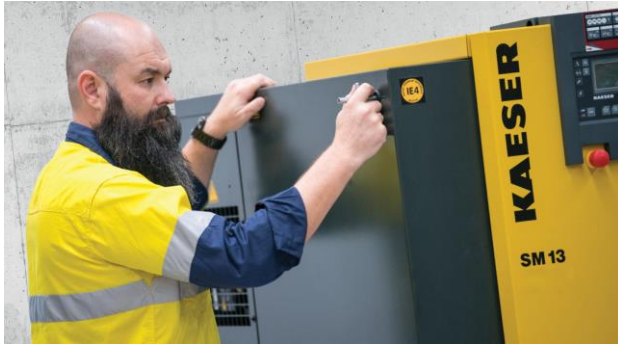
Caption: The festive shutdown is the perfect time to schedule in larger compressed air maintenance tasks.
