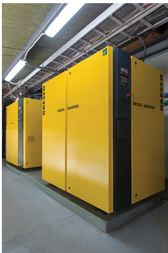
Caption: PSL installed a Kaeser CSD 105 rotary screw compressor and a Kaeser DN 22 series booster
