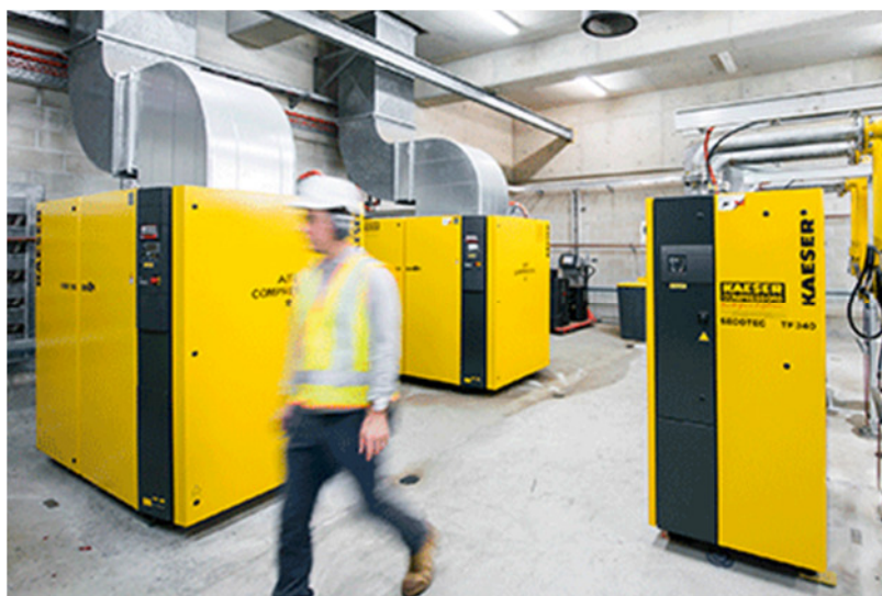
Caption: The upgraded compressed air system at Malabar Waste Water Treatment
