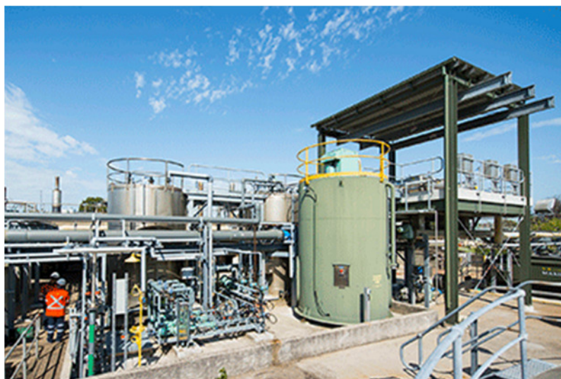
Caption: The Polymer system at Malabar WWTP, a part of the new sludge screening facility
